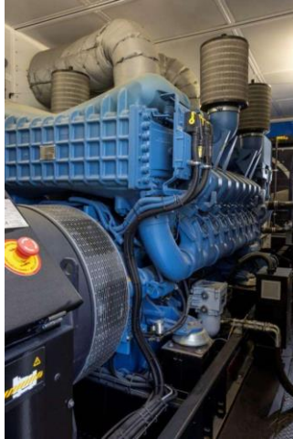
HIMOINSA generators to be installed on site - Credits: CoolPlanet
